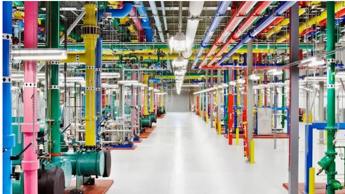
Data center cooling
